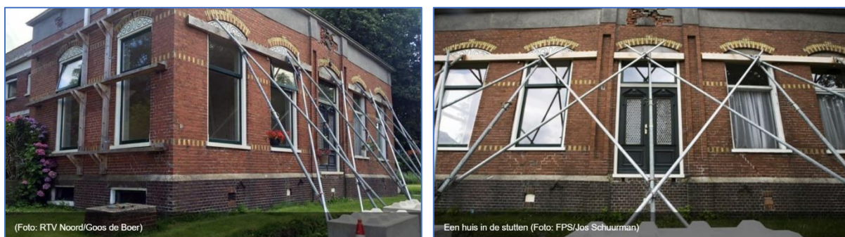
Figures 70. House in the struts/props with side view and front view. The large damage above the double door in the middle indicates a structural problem related to the high windows, narrow piers between the window frames and the distribution of the inner walls, with a lack of a continuous connecting diaphragm under the roof. These are architectural aspects from before 1920 and have nothing to do with inherent defects, because that was how people built at the time.
