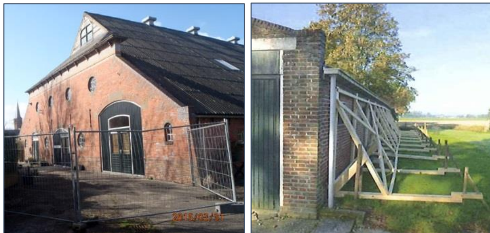
Figures 51. Left. Barrier around a high-risk facade construction. The flexible roof provides no support (but does provide additional load) on the already large mass of the high-top facade. Right: Struts of an old bad side wall.
