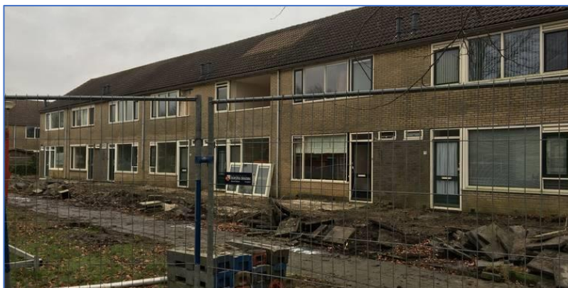
Figure 48. The suburb Opwierde-Zuid in Appingedam. Demolition of 233 houses for rebuilding. Photo: Gea v Loon, 9-1-2020. Dagblad v Het Noorden.
