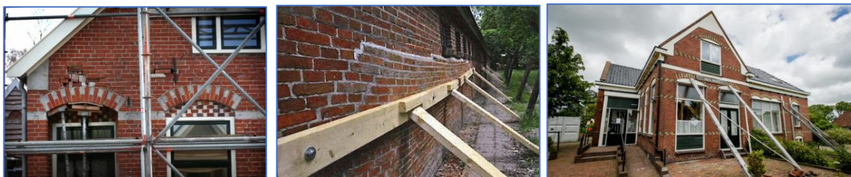
Figures 95. Different methods of shoring are used including scaffolding inside the buildings. Because of the publicity from these struts by the media, a lot of attention was paid to the buildings with these struts. 132
