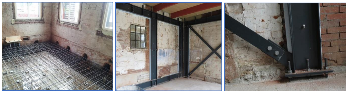
Figures 101. In some test houses, a full (reinforced) platform foundation and extra heavy inner and outer wall reinforcements and diaphragms were applied in 2015 to withstand a PGAg 0.36 according to the NPR9998:2015 map. These integral reinforcement operations on old buildings usually cost twice more than the value of the entire house.
