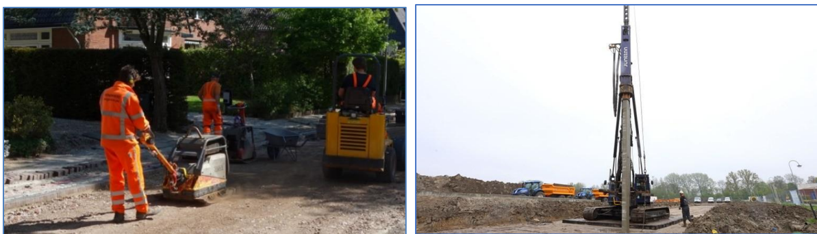
Figures 13. Due to the deep location, surface vibrations (bottom noise) are avoided. Soil compactor in the street. A piling installation can still be felt by people up to 500 m (photo Arcantus, Appingedam new construction).
